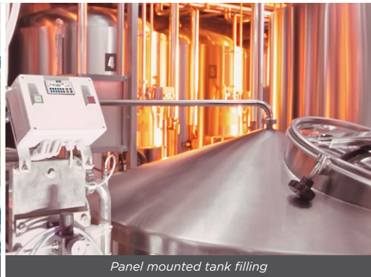
Panel mounted tank filling
